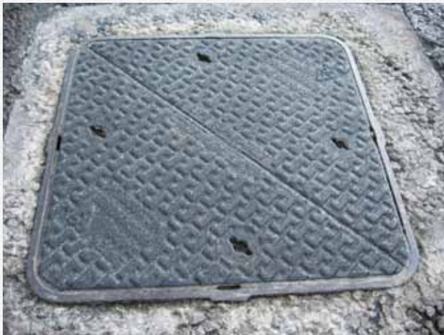
PREMARK® Anti-Skid securing man hole cover. Viaxi® primer enables good binding between the surface and the high friction material.
